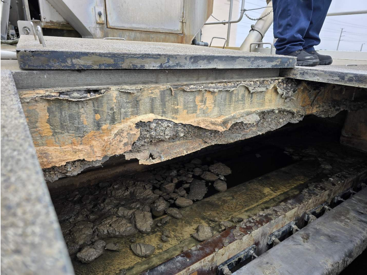
Figure 3-9 Photo 7 – Lining Failure at Concrete Beam
