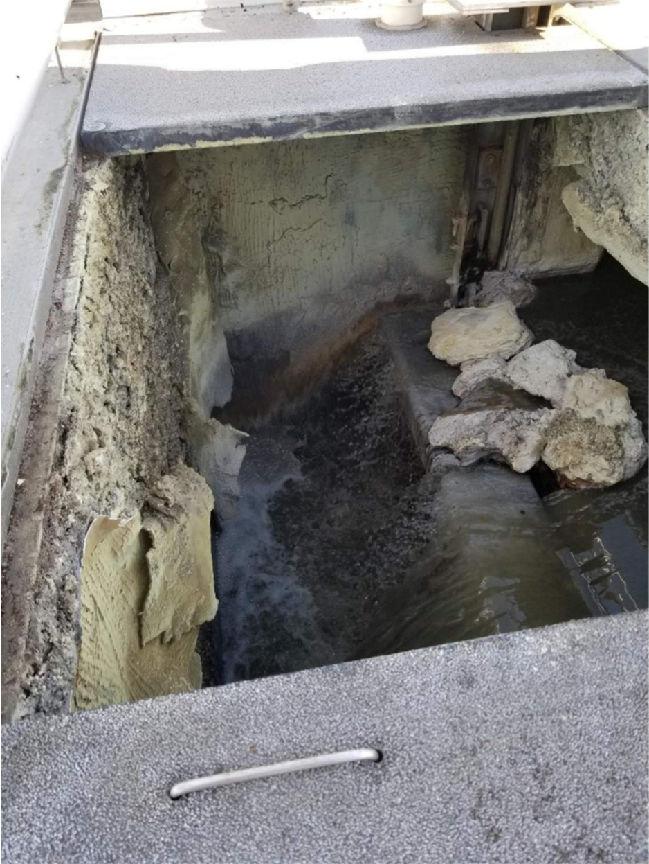
Figure 3-8 Photo 6 - Grease Accumulation at Weir Chamber
