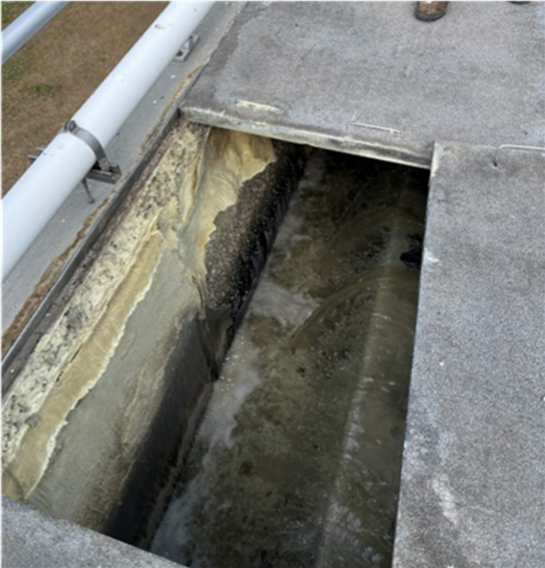
Figure 3-5 Photo 3 - Lining Failure at Weir Chamber
