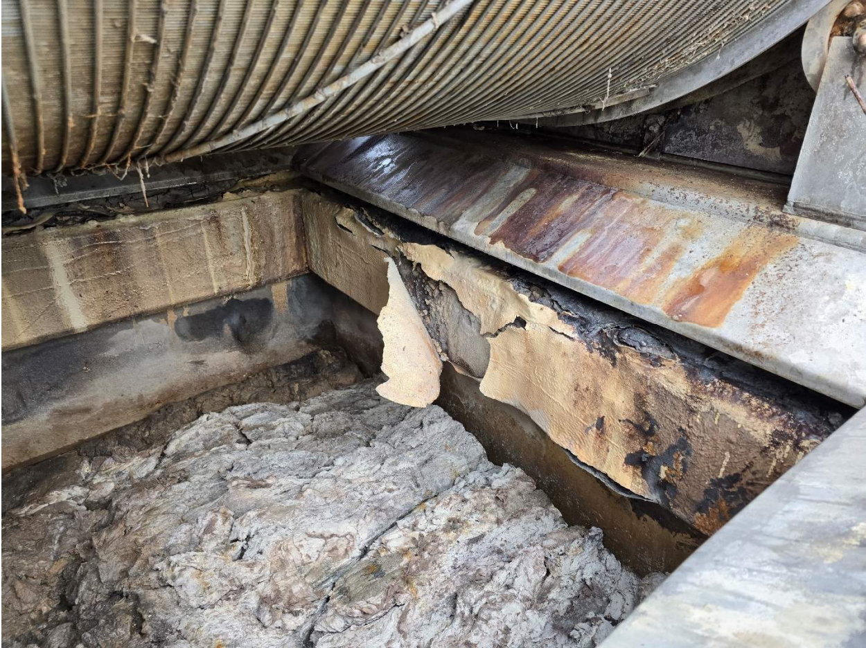
Figure 3-10 Photo 8 – Lining Failure Under Rotoshear Equipment
