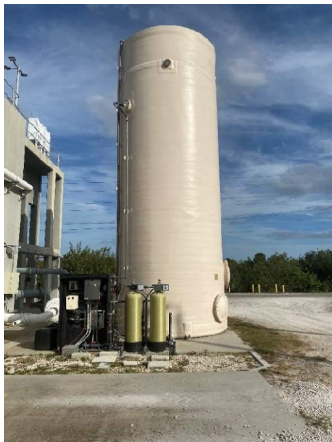
Figure 2-1 Existing Odor Control Unit at Headworks
