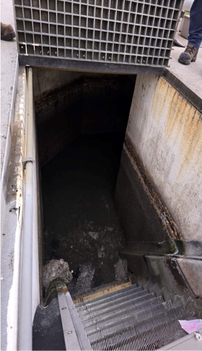
Figure 3-6 Photo 4 - Lining at Bar Screen
