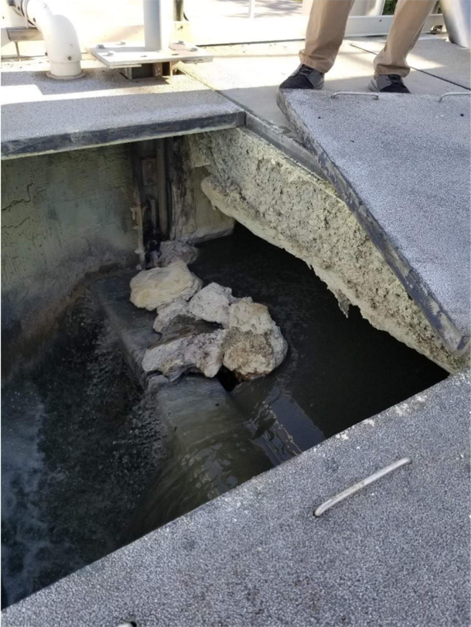
Figure 3-7 Photo 5 - Grease Accumulation at Weir Chamber
