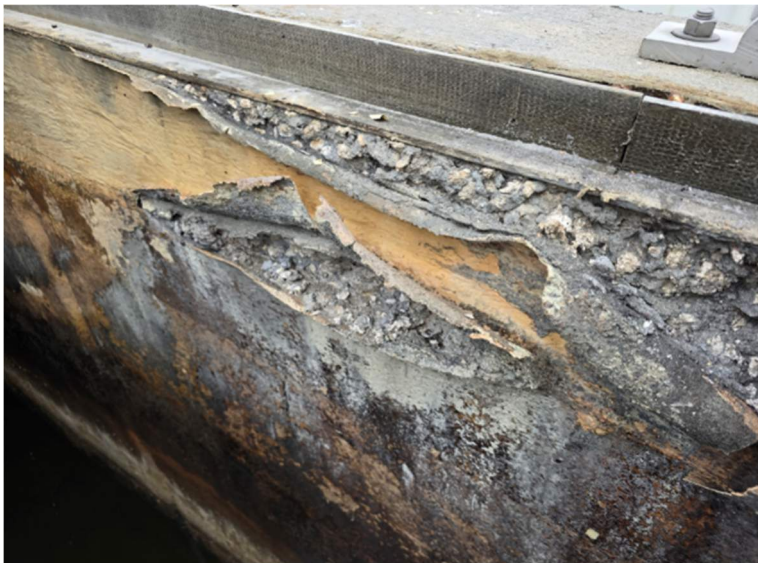
Figure 3-4 Photo 2 - Lining System Failure
