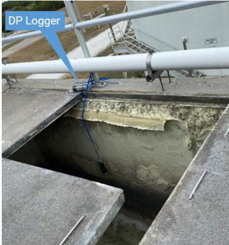
Figure 2-6 DP Datalogger at Headworks
