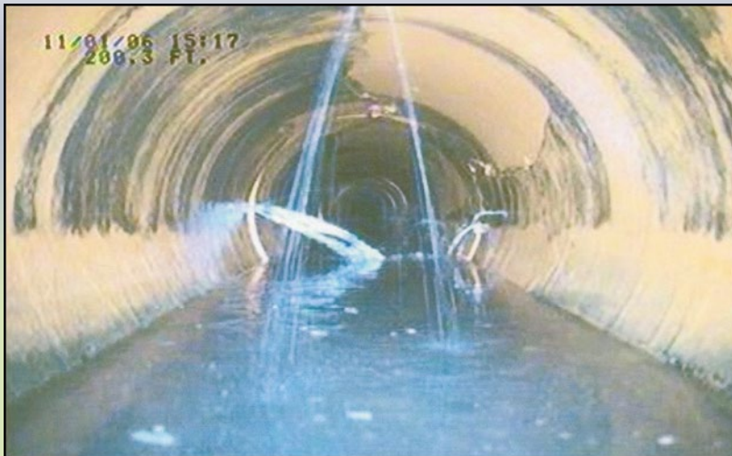
Figure 16 - Groundwater infiltration in sewer pipe
