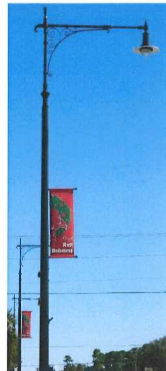
(Street lights installed in 2018 along US 192)
